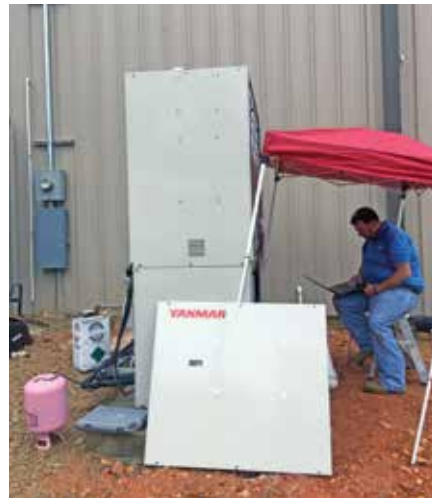
The Yanmar Co. Ltd. chiller provided an office in Alabama with lower utility and maintenance costs, quieter operation and reduced environmental impact through the use of clean-burning natural gas.
