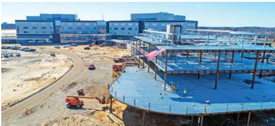
Inspira Medical Center Mullica Hill in southern New Jersey is installing a new natural gas-fired CHP system that will save the campus $1 million per year in energy costs.
