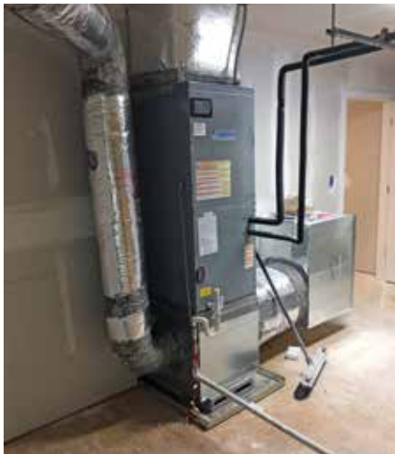
The STAE group of contractors deployed one, 12-ton natural gas-powered, VRF system which was connected to three 4-ton air handlers for both heating and cooling.
