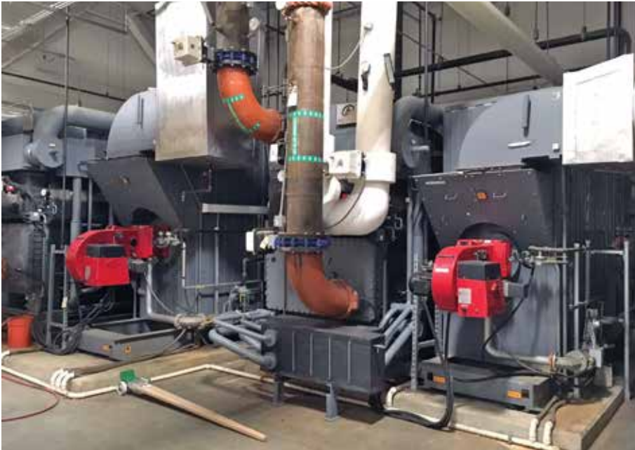
The Jordan Furniture facility is cooled and heated by 739-ton and 537-ton, direct-fired absorption chillers by Broad U.S.A. that burn natural gas and convert it to chilled water for air conditioning.
