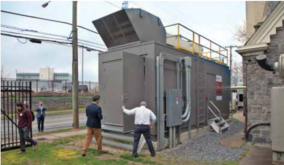
Cathedral Village replaced failing equipment with a high efficiency 265 kW natural gas engine by ENER-G Rudox to provide heat and electricity.
