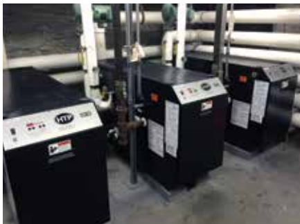
Manufactured by Emerson Swan, a local manufacturer, the modular boiler system at The Providence Center operates at 94 percent efficiency.
