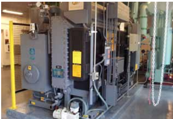
Sempra's corporate learning center uses Broad USA's absorption chillers to provide energy for its chilled, hot and domestic hot water plant.
