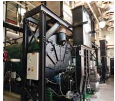
Nestle Purina PetCare in St. Louis replaced its trio of 45-year-old 300 HP steam boilers with two high-efficiency 500 HP boilers.
