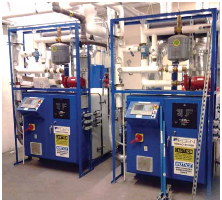
Multiple 70 kw CPH units help to power downtown Philadelphia high rise buildings while providing heat and hot water for commercial and residential tenants.
