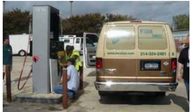
Engineers and technicians perform a final check of the new CNG dispenser just prior to becoming operational for McShan Florist. Bruce McShan can now refuel his fleet of 25 Ford E-350 vans onsite. The station opened to the public on October 26, 2012.
