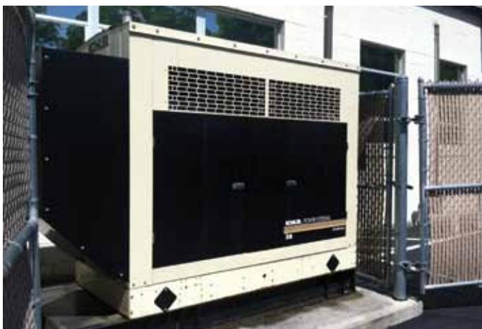
For Richards Mobil gas station in South Glastonbury, Conn., this backup generator made the difference between staying afloat and losing both sales and inventory when Superstorm Sandy hit in October 2012.
