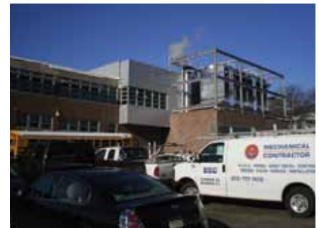
Becton High School in East Rutherford, N.J. replaced its electric boilers with a combined cooling, heat and power (CCHP) system using gas chillers from Broad U.S.A. Inc.
