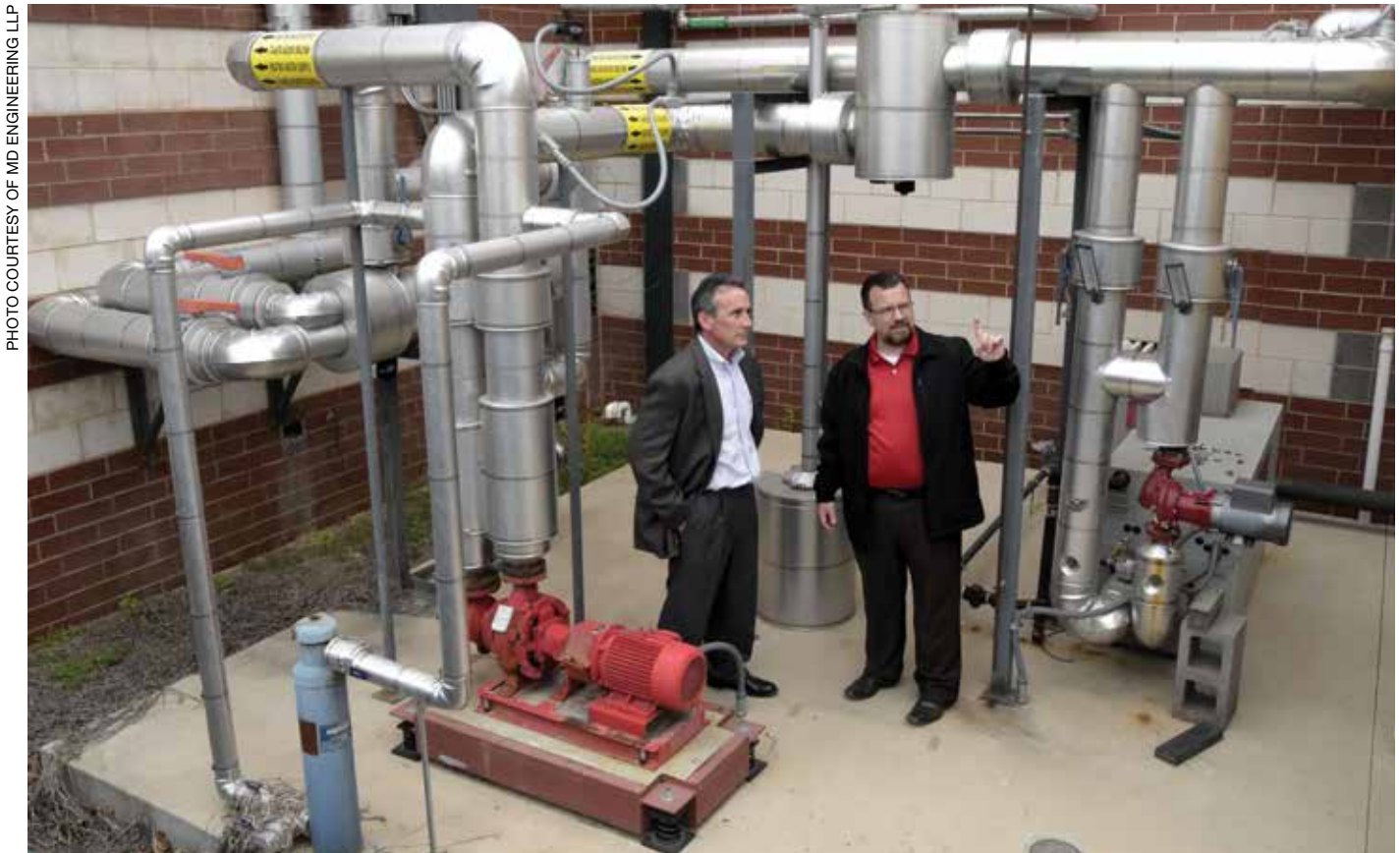
Greg Anderson (left), commercial marketing manager, Atmos Energy Inc., and MD Engineering President Michael Smith inspect the combined heat and power (CHP) system at the Oak Point Recreation Center in Plano, Texas. Smith designed the unit, which provides power for operating the facility's constant electric load as well as heat for maintaining consistent 84-degree water temperature in the center's large swimming pool.
