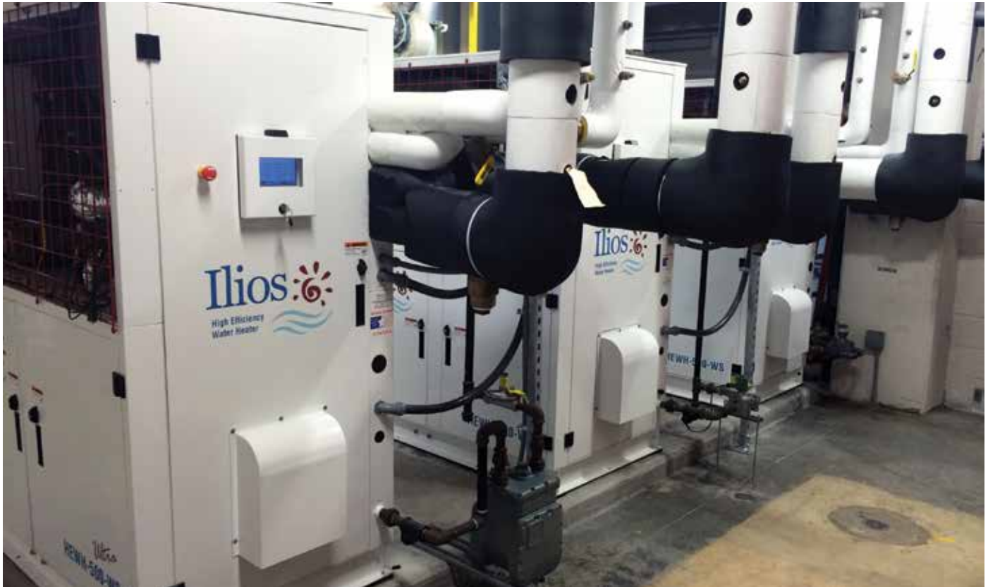
PHOTO COURTESY OF TECOGEN INC.
