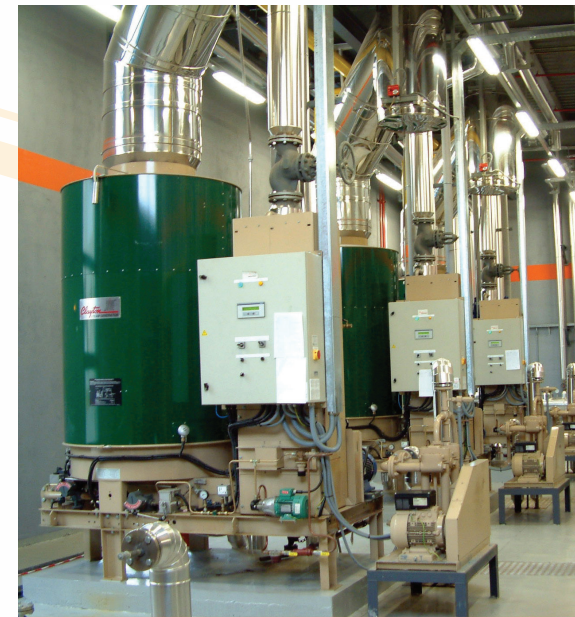
Vertical boilers are well-suited to modular boiler arrangements. Here are three 500 bhp units that serve a pharmaceutical plant. Compact size allows space for future boiler additions as needed. Courtesy: Clayton Boilers.
