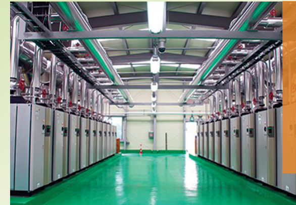
An example of a large number of compact boilers giving great flexibility and system redundancy. A digital control system manages boiler duty hours and optimizes units for peak efficiency. Courtesy: Miura Boilers.
